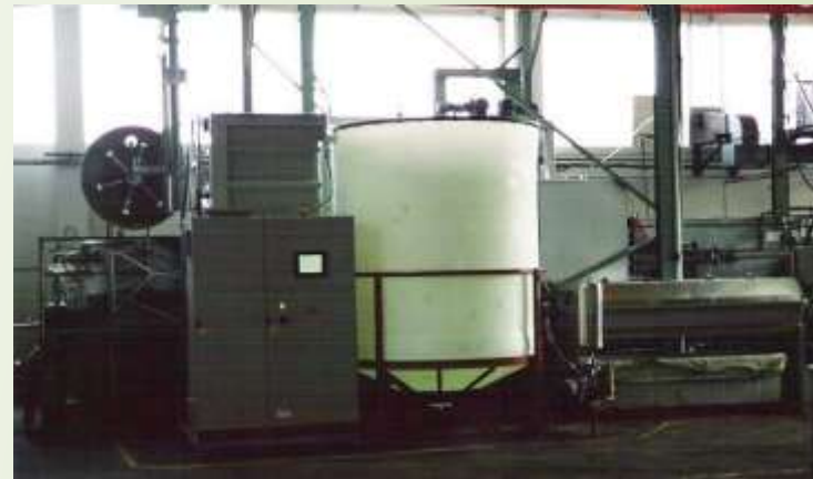
Water recirculating plant from impregnating process LOCTITE®, installed and running since 1995 in Sala Bolognese (BO) c/o MARTINI & C. S.r.l.
