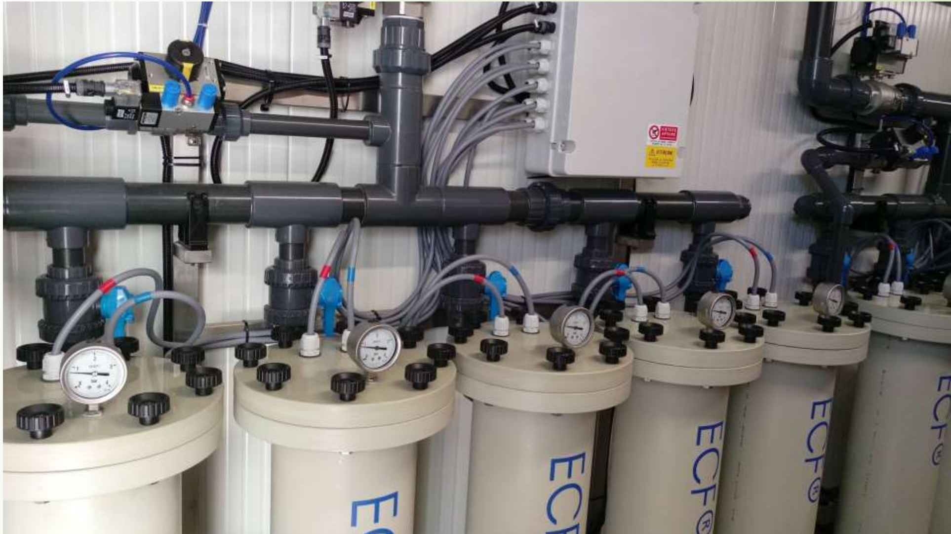
ECF Container - Tanning wastewater
