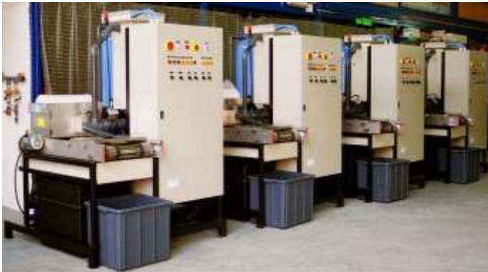
First series of water recirculation systems from Vibro finishing waste water -1992
