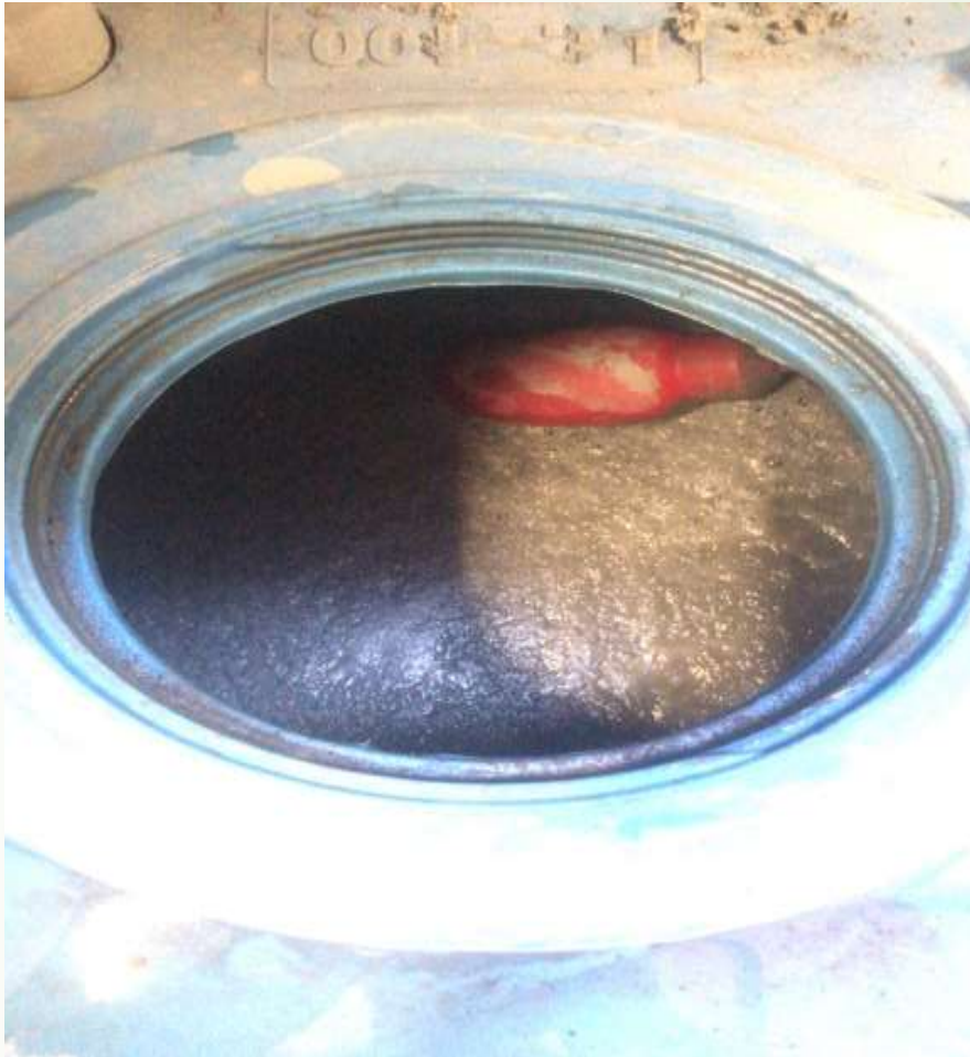
RAW EFFLUENT TANK – LOOK OF EFFLUENT QUALITY
